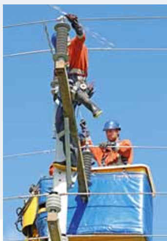
Winton-Hedgehope 66kV subtransmission line
