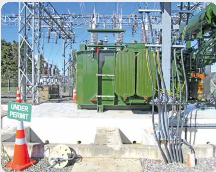
Ohai zone substation
