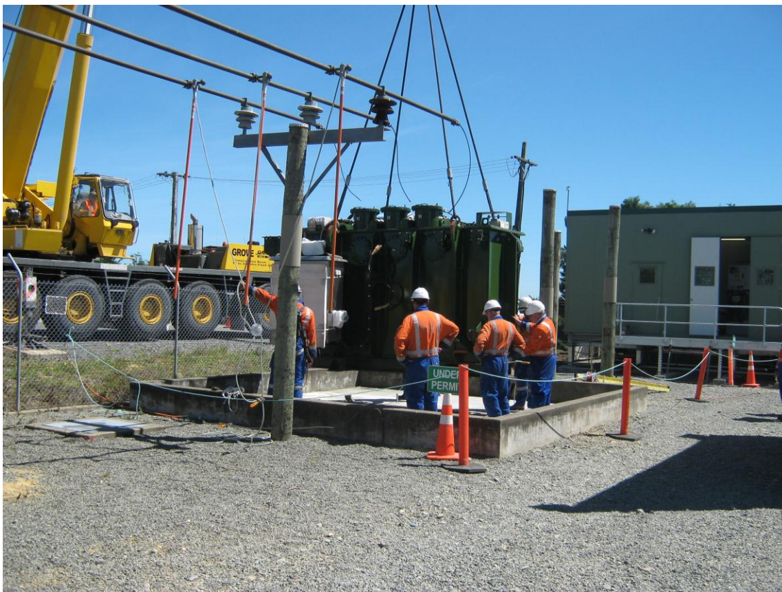
One of the two new 33/11kV transformers being lifted into place at the Kennington Substation.
