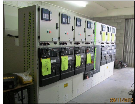
New switchboard at South Gore Sub
