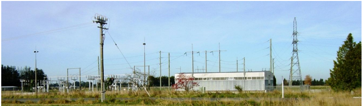
Figure 1 - Winton 66kV Substation
