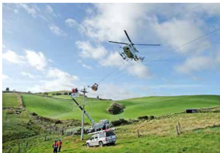
A helicopter assisted in the 33kV line rebuild between Kaka Point and Owaka
