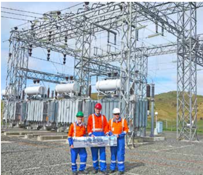
(L to R) Terry Jones and Bevan Cooper (PowerNet) with Don Simms (Transpower) at the Palmerston Substation
