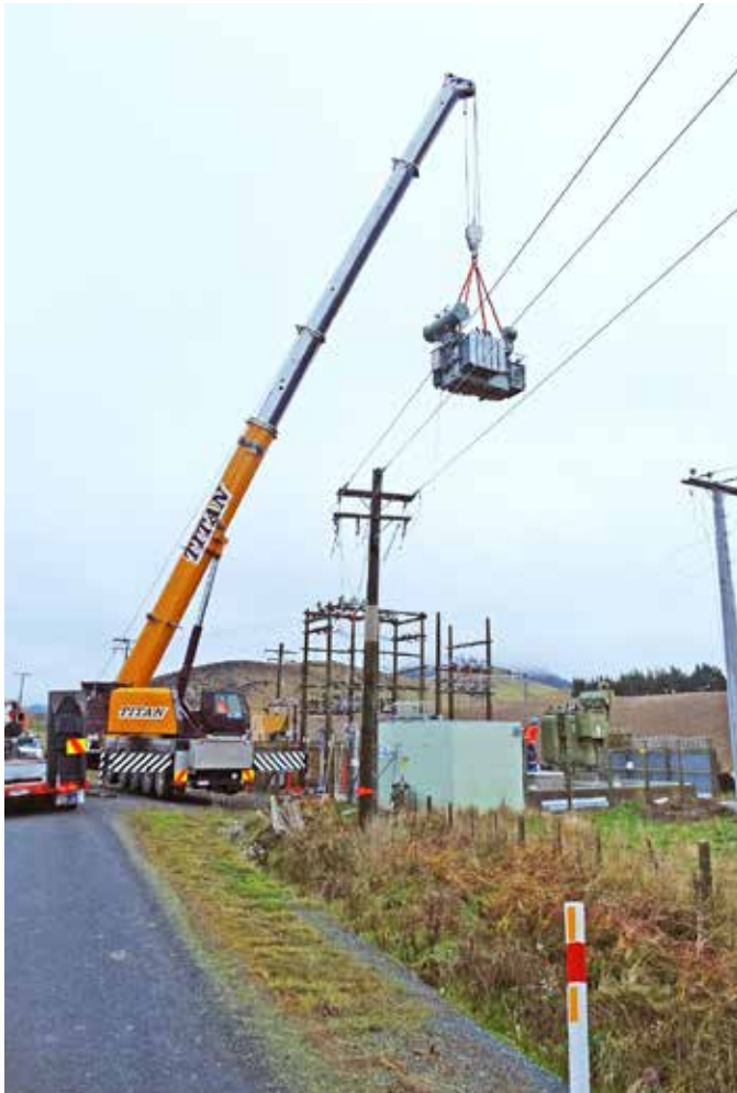
The 14.1 tonne transformer being lifted over the 11kV lines onto the Clinton Substation site
