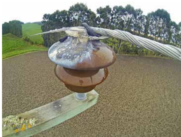
This photo shows damage to an insulator caused by the extreme heat of an electrical fault. This fault and arc may have been started by some foreign material (e.g. a branch) or a lightning strike. An electric arc is when the electricity jumps across a gap rather than going through the wires
