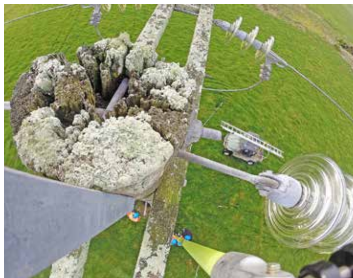
This photo is looking at the split head (top) of a pole. The GoPro camera has been attached to the yellow insulated stick and elevated allowing the pole to be inspected
