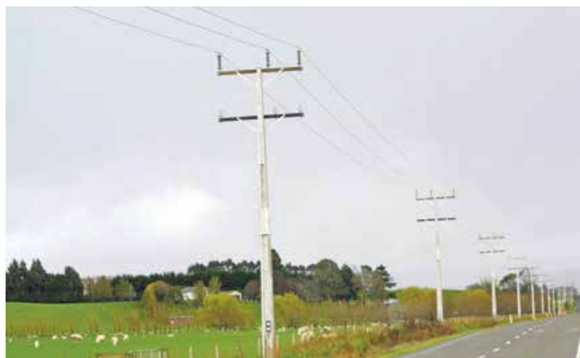
Fairfax to Isla Bank 66kV line
