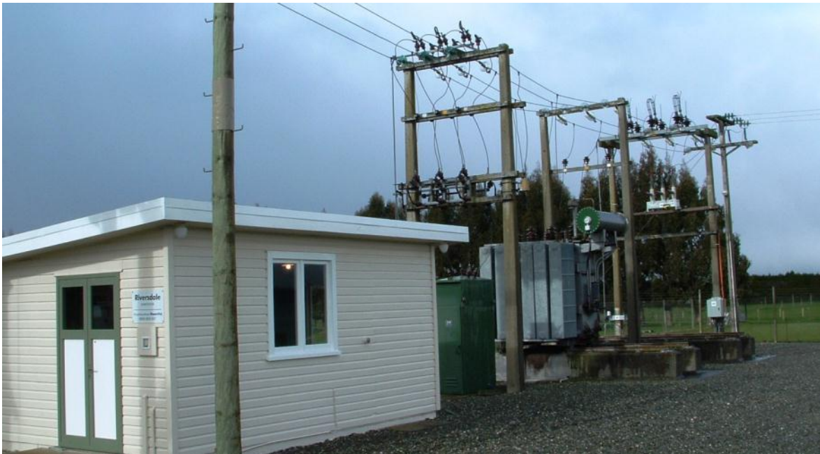
Figure 46 - Present Riversdale substation
