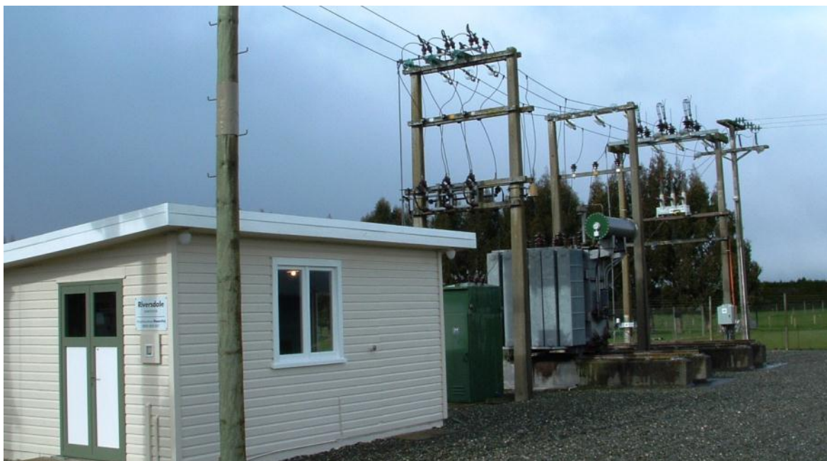
Figure 3 - Present Riversdale substation
