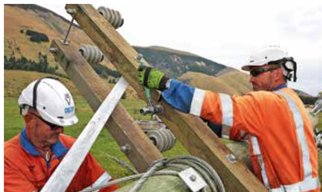
Delta line mechanic brothers Vince and Marcel Moore preparing poles to be erected on stage 3 of the Mossburn to Athol line upgrade
