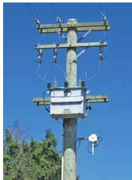
An installed relay unit (lower right) on The Power Company network
