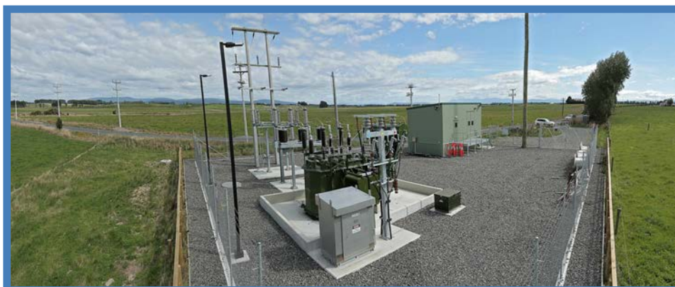
Photo: Isla Bank Substation
