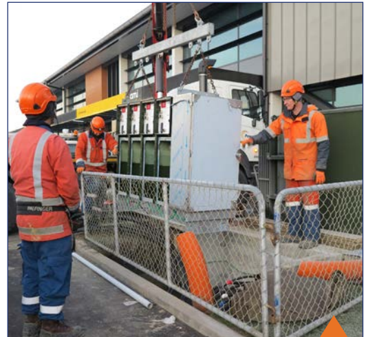
Left to Right - PowerNet's Jordan Coutts, Andrew King and Paul Barclay, lifting the new switchgear into position at sub 519
