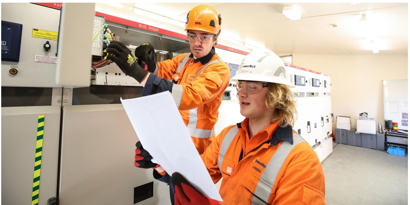
Aaron McCallum and Joseph Wynne working on the protection upgrade at Edendale Zone Substation.
