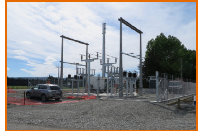
Top: PowerNet's mobile substation.
