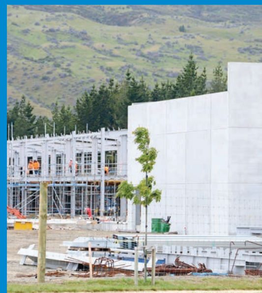
Work commences on the project to construct the new Wakatipu High School
