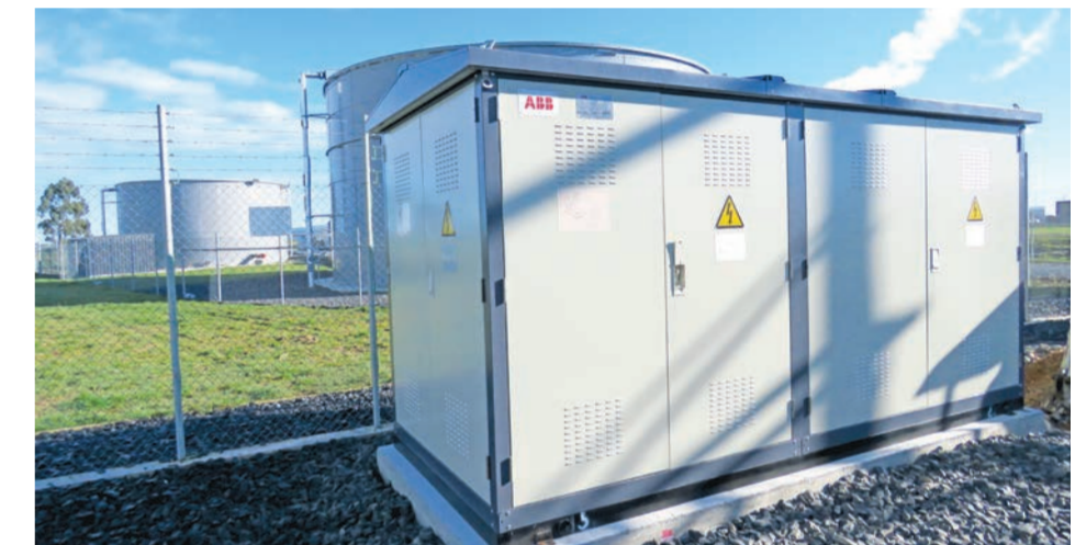
The weatherproof housing for the indoor 33kV Ring Main Unit
