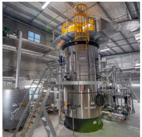
The 13MW electrode boiler at Open Country Dairy in Awarua.
