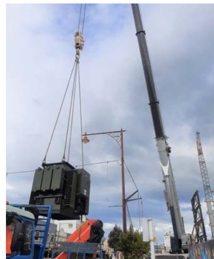
One of the two 1.5MVA transformers being positioned into Invercargill's CBD development site.
