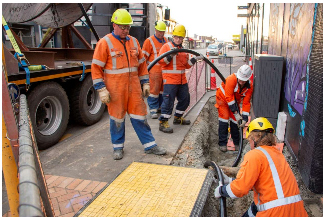
PowerNet and BCL pulling new cables to upgrade the network for the Langlands Hotel complex
