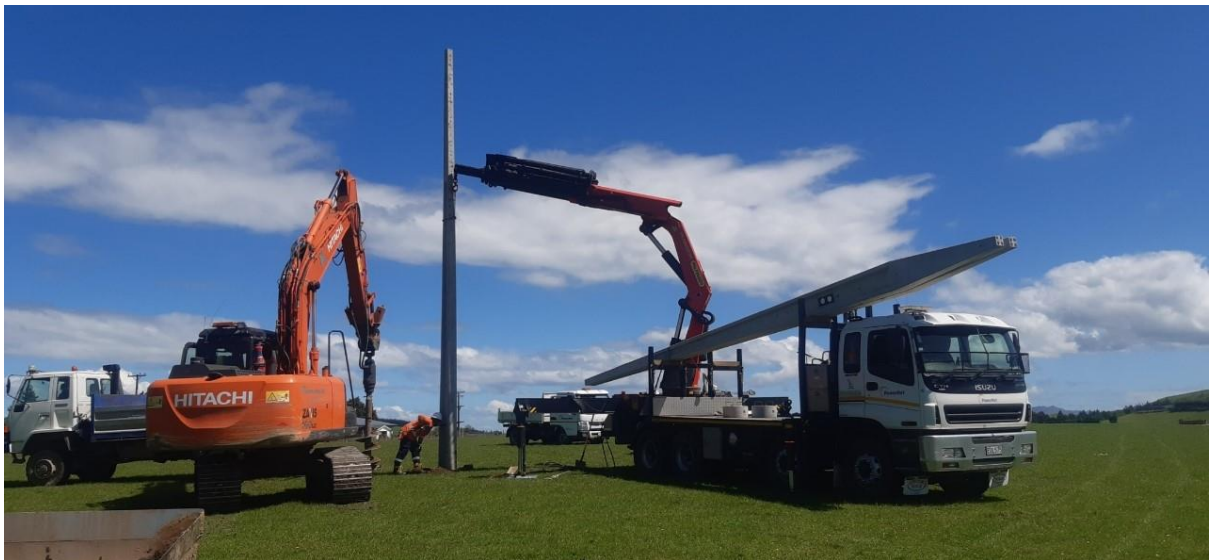
The Gore PowerNet team installing the first 33kV pole at the Kaiwera Downs Wind Farm site
