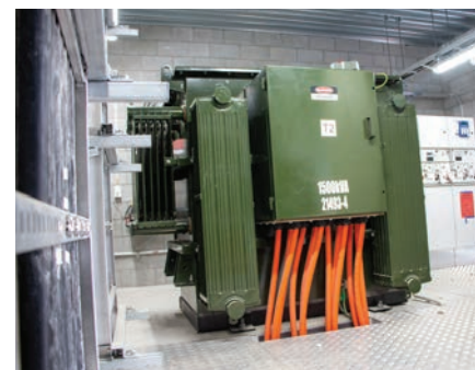
One of the two 1.5MVA transformers at the Invercargill CBD development.
