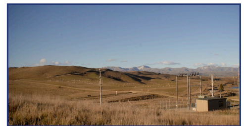
OtagoNet's Waipiata Zone substation.
