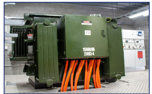
One of the two 1500kVA transformers supplying the Invercargill Central Mall.
