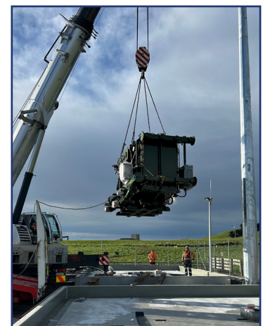
The first 25MVA transformer being installed at the McNab substation on the outskirts of Gore.
