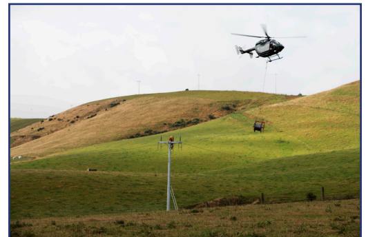
Contractor, Otago Helicopters, stringing the conductor onto the 171 poles and supporting structures across the 14.5 km overhead route as part of Mercury Energy's 43MW Kaiwera Downs Wind Farm project.
