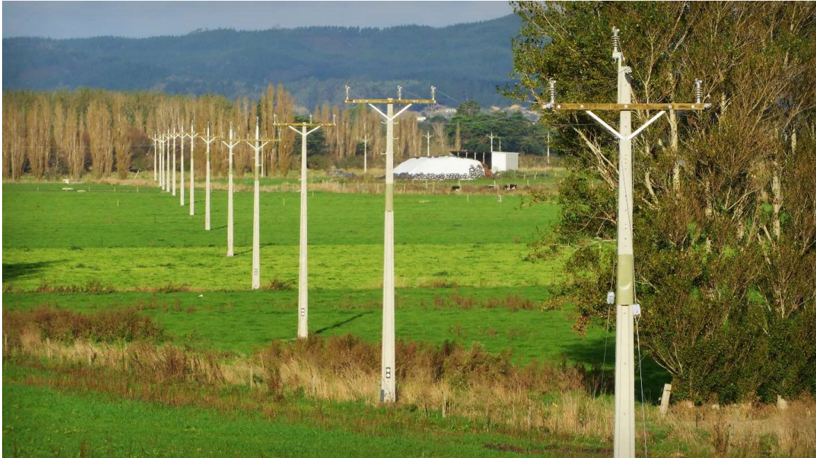
The 33,000 volt power line to Kaitangata, rebuilt in 2022/23
