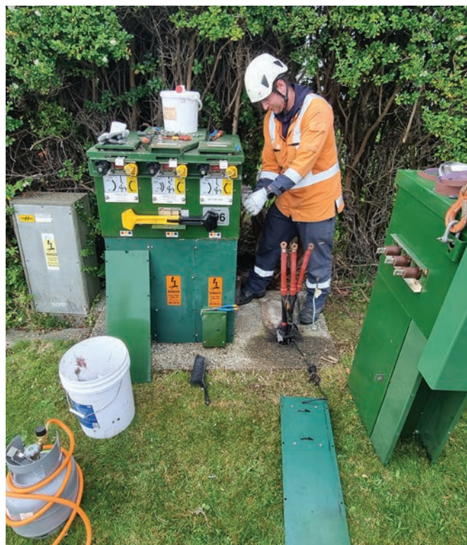
Ring main unit maintenance on the EIL network.
